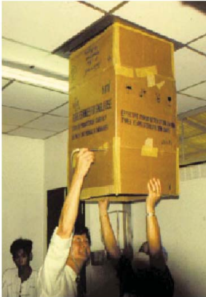
Using a carton box and flow velometer to monitor air flow in TB patient isolation room with mechanical ventilation system, Chiang Rai Hospital, Chiang Rai, Thailand
