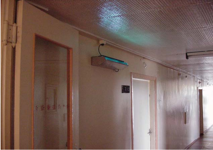
Picture 5: Upper air radiation with shielding placed below the UVGI source.
